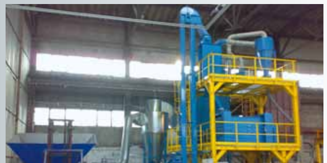
Screening technology featuring density sorting, conveyor technology and steel construction
