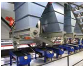
Screw conveyors, dosing tanks
